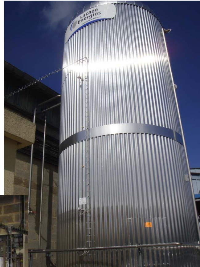
Thermal stratification tank
