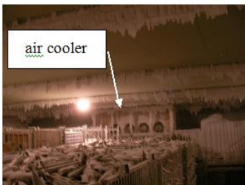
Figure 6 Existing ultra-low temperature refrigerator
