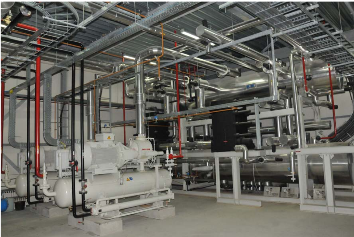
Figure 3: View on cascade NH 3 compressors & NH 3 /CO 2 vessel skids
