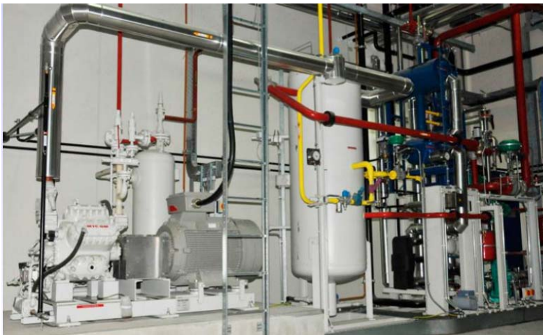
Figure 5 : View on hot water NH3 heat pump system
