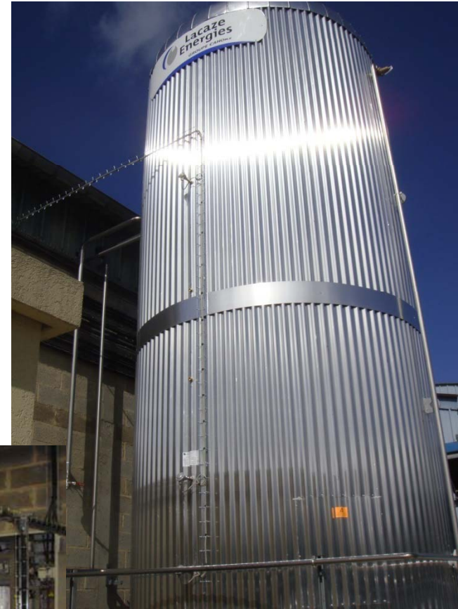
Thermal stratification tank
